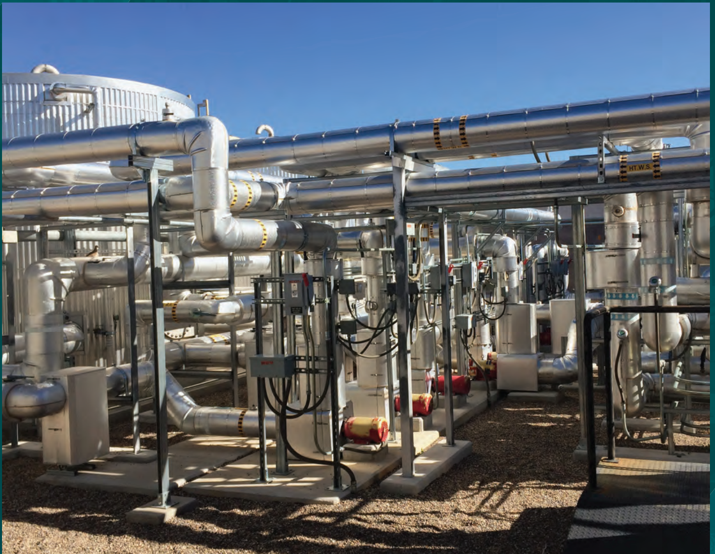
Pipes at the microgrid at Mesa del Sol.
