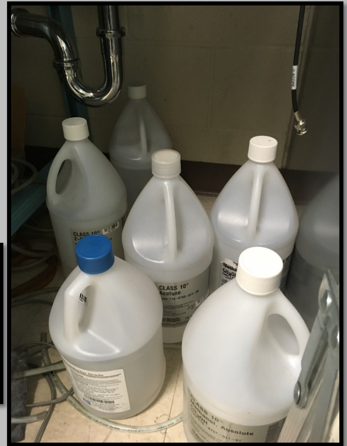
IMPROPER STORAGE – flammables stored under sink, on floor
