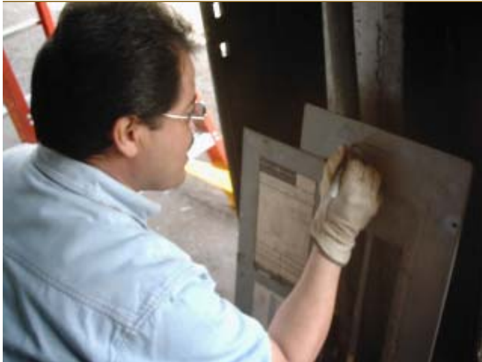
The Area Four electrical crew (Carlos Nevarez (pictured), Duane Stair, Donald Martinez, and Ralph Rodriguez) has been wiring the sheds and installing a power pole at the old Galles building for the engineering laboratories that will be relocated there. Carlos explains the safety procedures.
